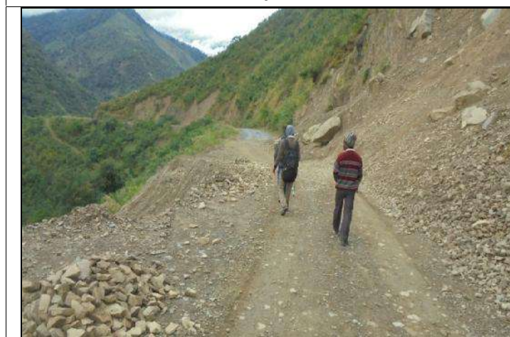
Sinking Zone at Ch. 12+500 km
