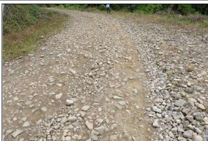
Poor Condition of Pavement
